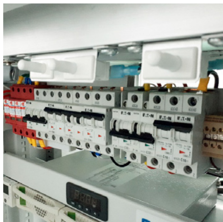
Painel de energia de cabine outdoor
